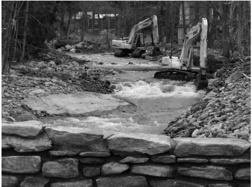
Excavators cleared the Konkapot River upstream of the Route 57 bridge in Hartsville
